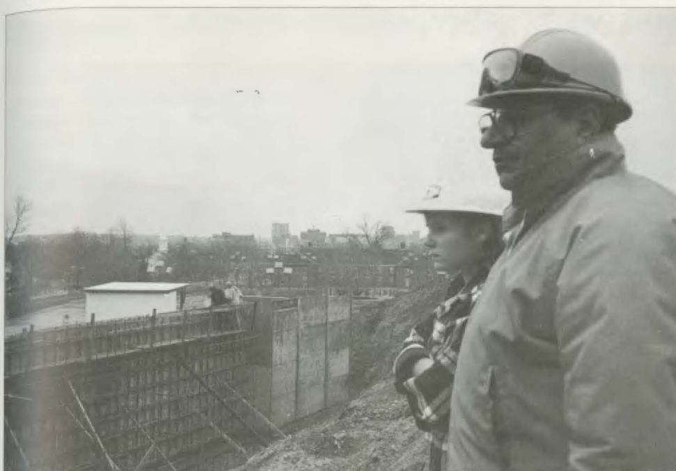
Jean Zukowski, engineer for Miller-Davis Construction, and John Kounelis, construction coordinator, inspect progress.
